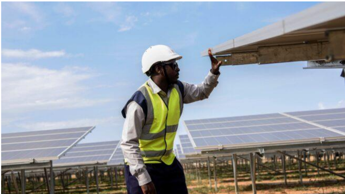
A maintenance engineer at a utility solar plant in Uganda. (Photo by Isaac Kasamani/AFP via Getty Images)
