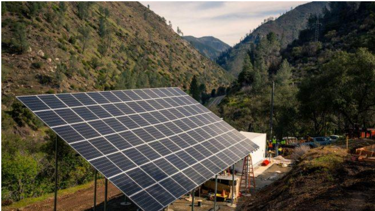
A stand-alone power system in Briceburg, California, with a solar photovoltaic array, battery energy storage system and backup propane generators. (Photo courtesy of BoxPower)
